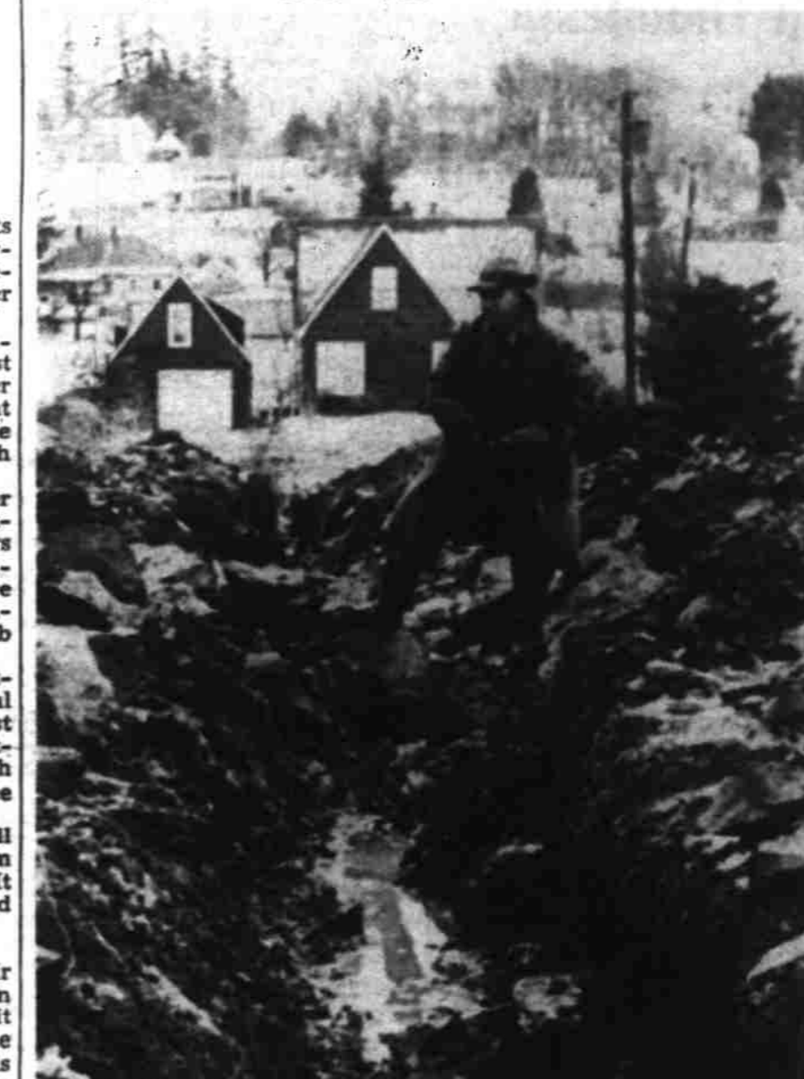
City water department crews blasting their way through rock for a new pipeline along East Nob Hill street in south Salem brought anxious queries this week to police and newspapers. Above is J. R. Rowland, 1854 State st., standing on one of the huge boulders which is plaguing workmen as they dig the ditch for a two-inch east iron main. To serve a new residential area, it will be supplied from an eight-inch line on Waldo avenue and will tie in to a stub-line at Ohmart street, extended from McElhrist st. (Statesman photo.)
