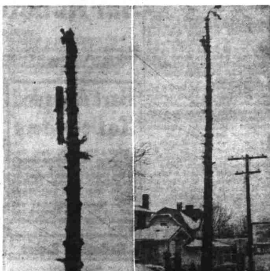
Down she goes... and as the top of a 100-foot fir tree topples, high climber Curly Davis, 753 S. 13th st., hangs on. The action took place Friday at 1249 S. Commercial street, home of H. A. Harrington, where the tree is being removed by John Brennan and Sons, tree surgeons. At right Davis is shown high up on the old fir preparing to saw off the top with an IEL power saw, an unusual procedure in topping. The tree, as with another removed three weeks ago, was endangering nearby buildings. (Statesman photo.)
