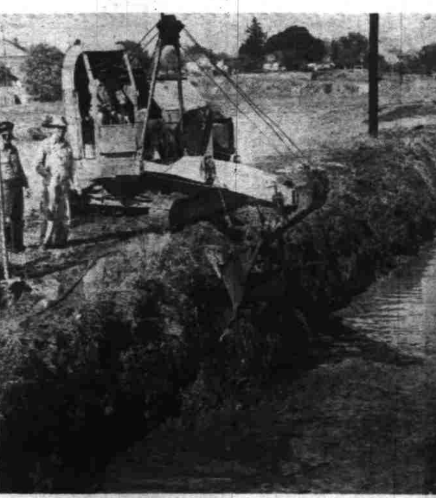
Junior high school and through Bush's pasture to Shelton ditch. At left is a shovel crew with, left to right, Arthur Robbins, 2846 S. Commercial st.; Foreman Vera Robbins, and shovel operator Tom Conyer, 2667 Portland rd.; and at right is a drag line operated by Harold Eckstein, Keizer. (Statesman photos.)
