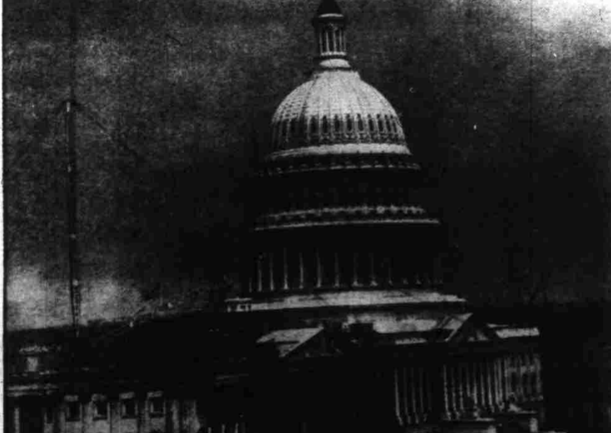
CAPITOL UNDERGOES REPAIRS —In midst of derricks and scaffolding, workmen repair Capitol roof at Washington. House and Senate chambers will be completed in December.
