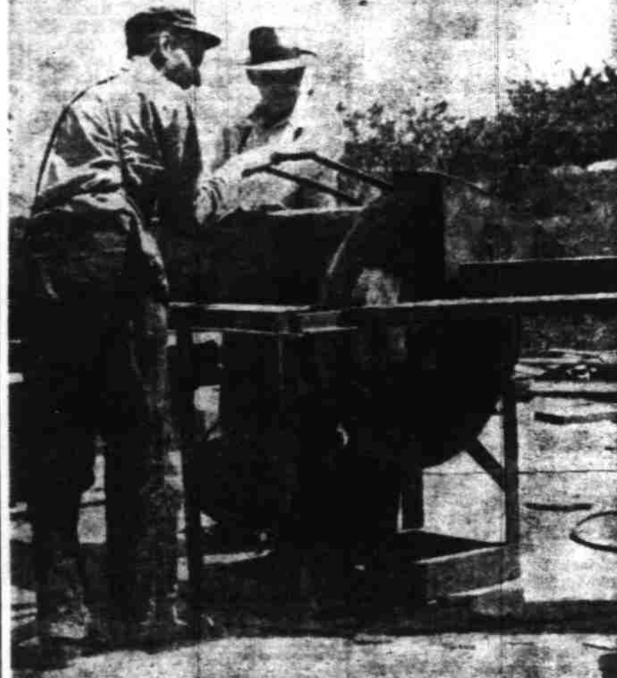
Specially planned and grooved logs are cut to size on the building site with power saws, as above. Operating saw is E. A. Roberts, Portland, who has been active in erecting log structures in Oregon, as C. W. Wright looks on. Above is a "Log Structure" house which was built in Canby.
