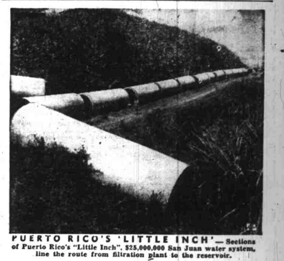
PUERTO RICO'S "LITTLE INCH" — Sections of Puerto Rico's "Little Inch," $25,000,000 San Juan water system, line the route from filtration plant to the reservoir.
