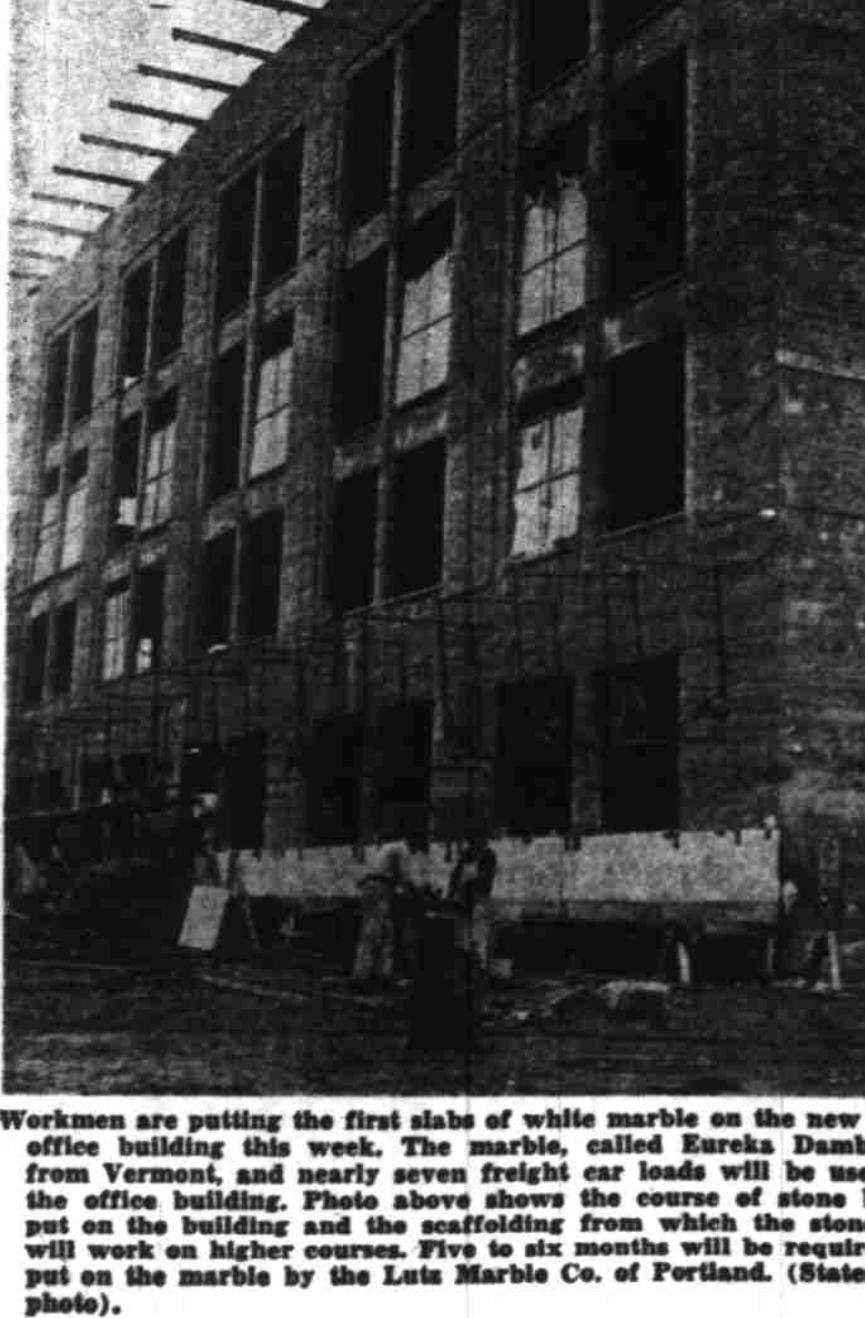
Workers are putting the first slabs of white marble on the new state office building this week. The marble, called Eureka Dumbo, is from Vermont, and nearly seven freight car loads will be used on the office building. Photo above shows the course of stone being put on the building and the scaffolding from which the stonemasons will work on higher courses. Five to six months will be required to put on the marble by the Lutz Marble Co. of Portland. (Statesman photo.)
