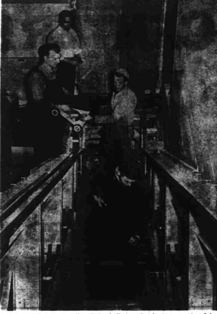
Riding platforms for the Robert Bros. store's new motor-driven stairs are being installed this week and will be ready for use by the end of this month. Manufactured by the Motorstair Co., of Coffeyville, Kans., the conveyance is being installed by H. J. Hanson, foreground; E. A. Lindblom, left center; H. J. Clow, right center; all of Seattle, Wash., and J. E. Ross, supervisor, Coffeyville, Kans., background. (Statesman photo).
