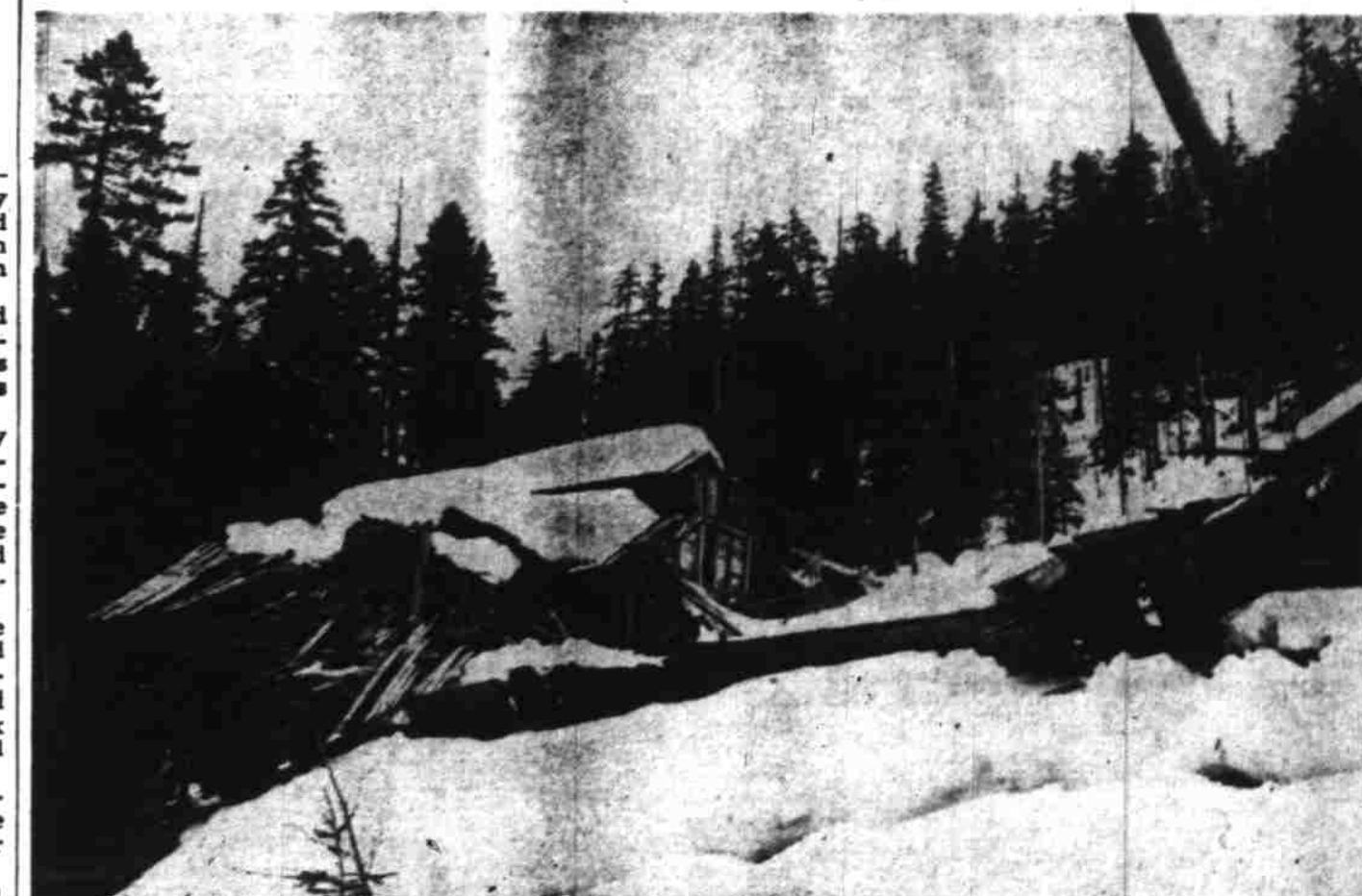
ELKHORN, March 3—This snow-covered wreckage is what heavy snow and storm left of the Pacific Smelting and Refining company's pilot mill which J. P. Hewitt used in development of huge zinc and lead deposits on his property 11 miles above here. The heavy snow marooned five miners and one woman in camp here until a rescue party arrived Wednesday.
