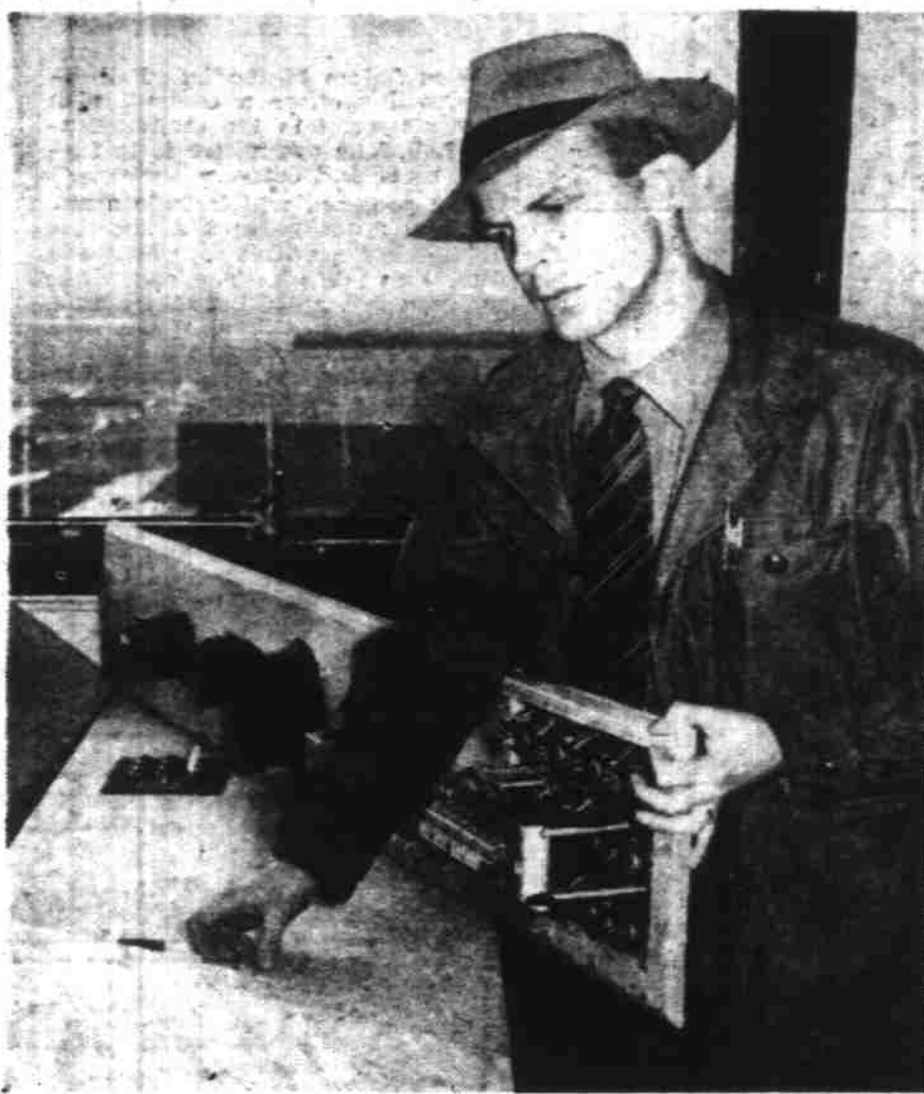
Radio facilities and office equipment are being installed in the air traffic tower this week as preparations are being made for its use at Salem airport. Shown above is W. E. Chambers, Seattle, Wash., civil aeronautics authority technician, at work on an instrument panel in the control room of the tower. Just when the tower will be ready for operation is not yet definitely known, being dependent upon arrival of all the radio and power equipment. (Statesman photo).
