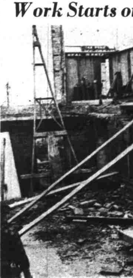
Steel beams for vertical support of a new building to be erected on the site of the burned-out Guardian building are shown above being slid into place Tuesday. Construction of the one-story store building will begin as soon as foundation and beams are ready. Vlesko & Post has the contract. (Statesman photo).
