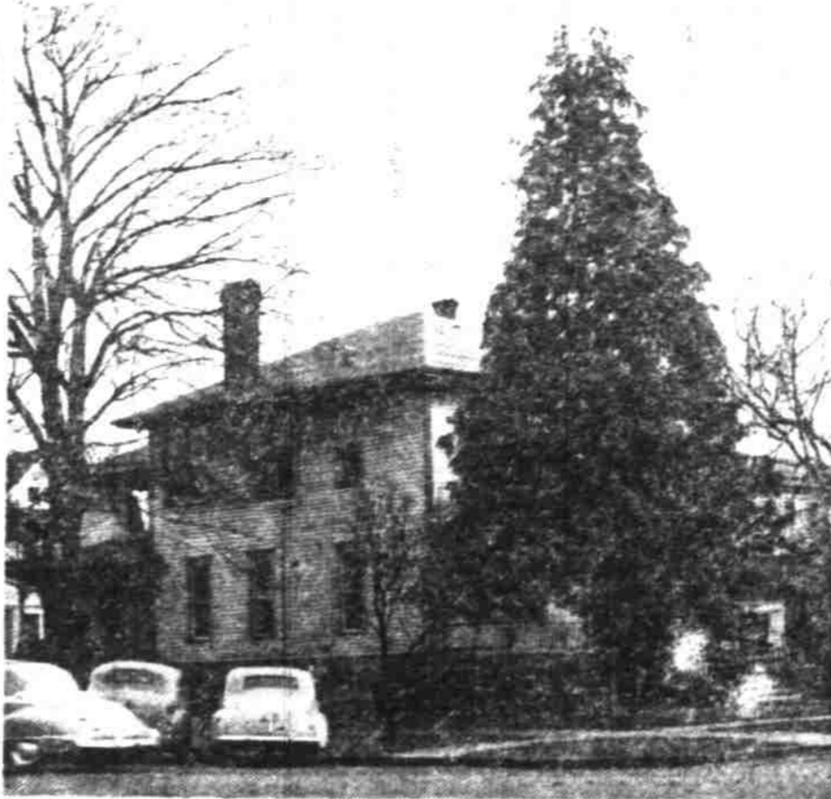
Now being razed is this historic house at the southeast corner of Chemeketa and North Church streets, where it is planned eventually to build the new home of The Statesman Publishing company. The house, until recently the F. G. Delano residence, is more than 80 years old. (Statesman photo).
