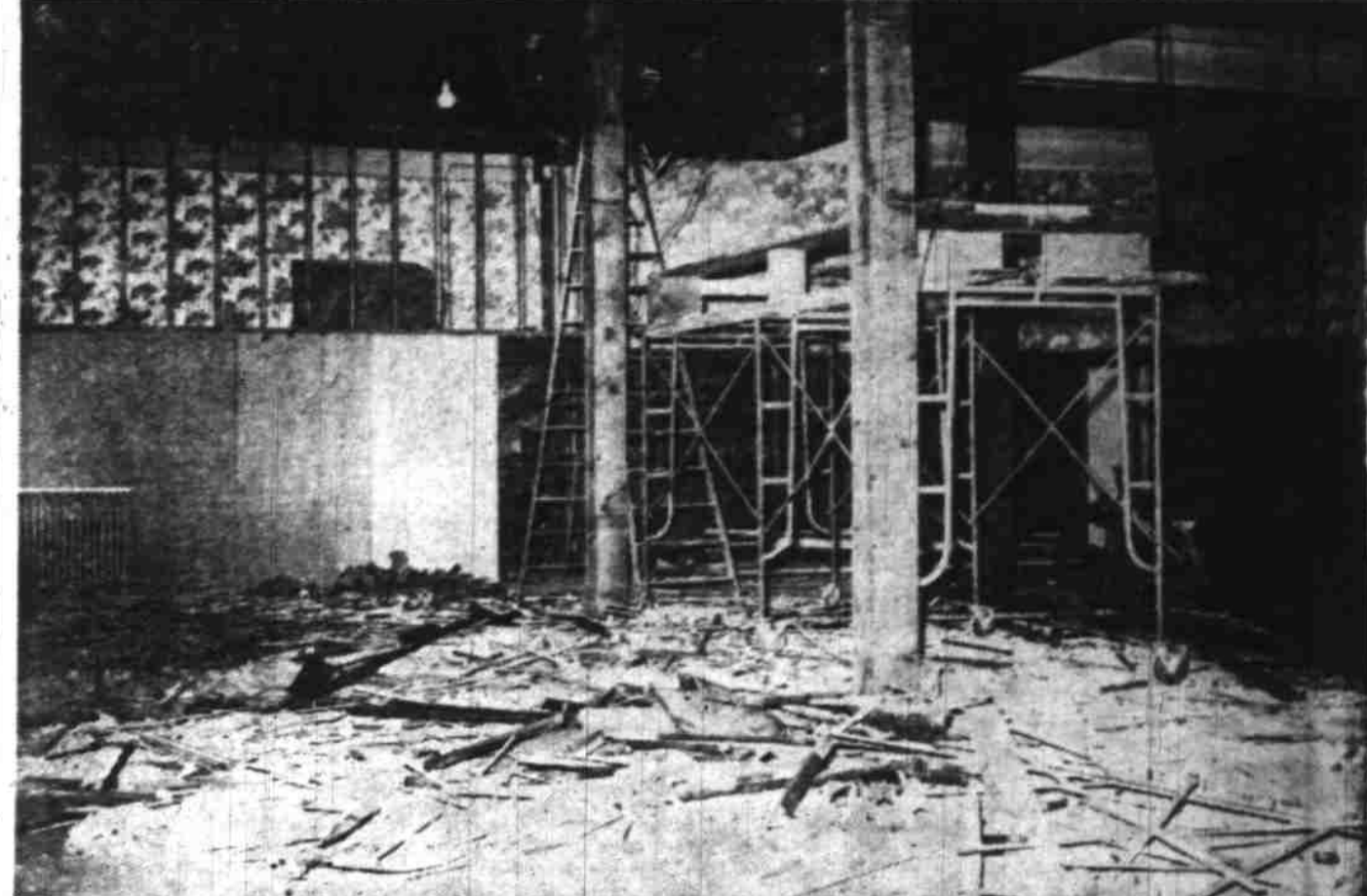
Marion hotel's historic "Mirror Room," meeting place for many of Salem's social and civic functions and scene of numerous legislative caucuses, will soon be minus its mirrors and posts. The photo shows the banquet hall in the process of a thorough renovation. Steel "T" beams will replace the posts which once supported roof and the room will be completely modernized and enlarged to handle larger crowds. Mirrors are already out. G. Clerico, hotel manager, said the job would probably be completed by early January before the 1949 legislature convenes. (Photo by Don Dill, Statesman staff photographer).
