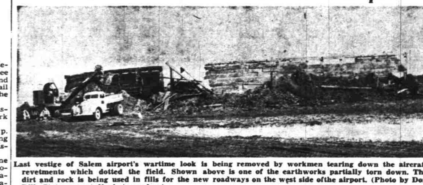
Last vestige of Salem airport's wartime look is being removed by workmen tearing down the aircraft revetments which dotted the field. Shown above is one of the earthworks partially torn down. The dirt and rock is being used in fills for the new roadways on the west side of the airport. (Photo by Don Dill, Statesman staff photographer.)
