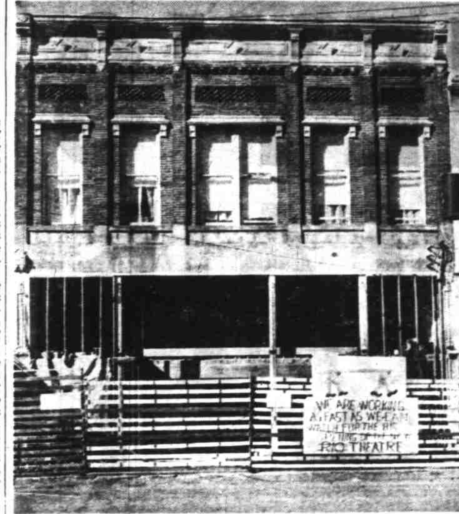
DALLAS—Complete remodeling of the Rio theater in Dallas will be finished early in November with major work being done from the foundations up. Shown above is the front of the old theatre building which will have a large, modernistic marquee. Donald E. Wernli, manager of the Rio and Majestic theatres, both owned by the Jesse Jones theatres of Portland, said that the new Rio will have new seats, decorations, screen and sound and projection equipment, and that it will seat 400 people. (Photo by Don Dill, Statesman staff photographer.)
