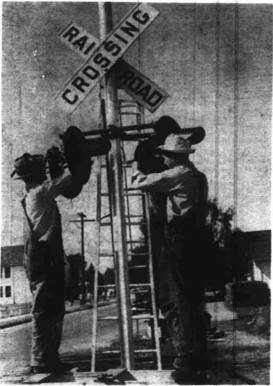
Installation of automatic warning signals is almost complete at the D street crossing of the Southern Pacific railroad, near Salem High school, after several weeks of work on the poles and relays. Shown above installing the lights on one of two poles are, left to right, T. V. Engle, Woodburn, and M. C. Miller, 1884 State st. The signals consist of four powerful red lights on each of the two poles. (Photo by Don Dill, Statesman staff photographer)
