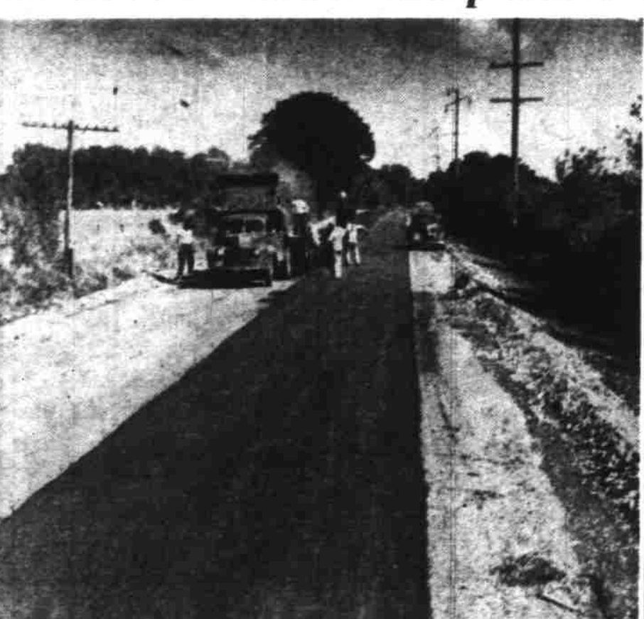
Fair weather Monday made possible completion of laying the base for a new strip on the Salem-Silverton highway between Middle Grove school and the Pudding river bridge, about 5.4 miles long. Two miles of topping and building of shoulders will be finished in a week if the weather holds. (Photo by Don Dill, Statesman staff photographer.)
