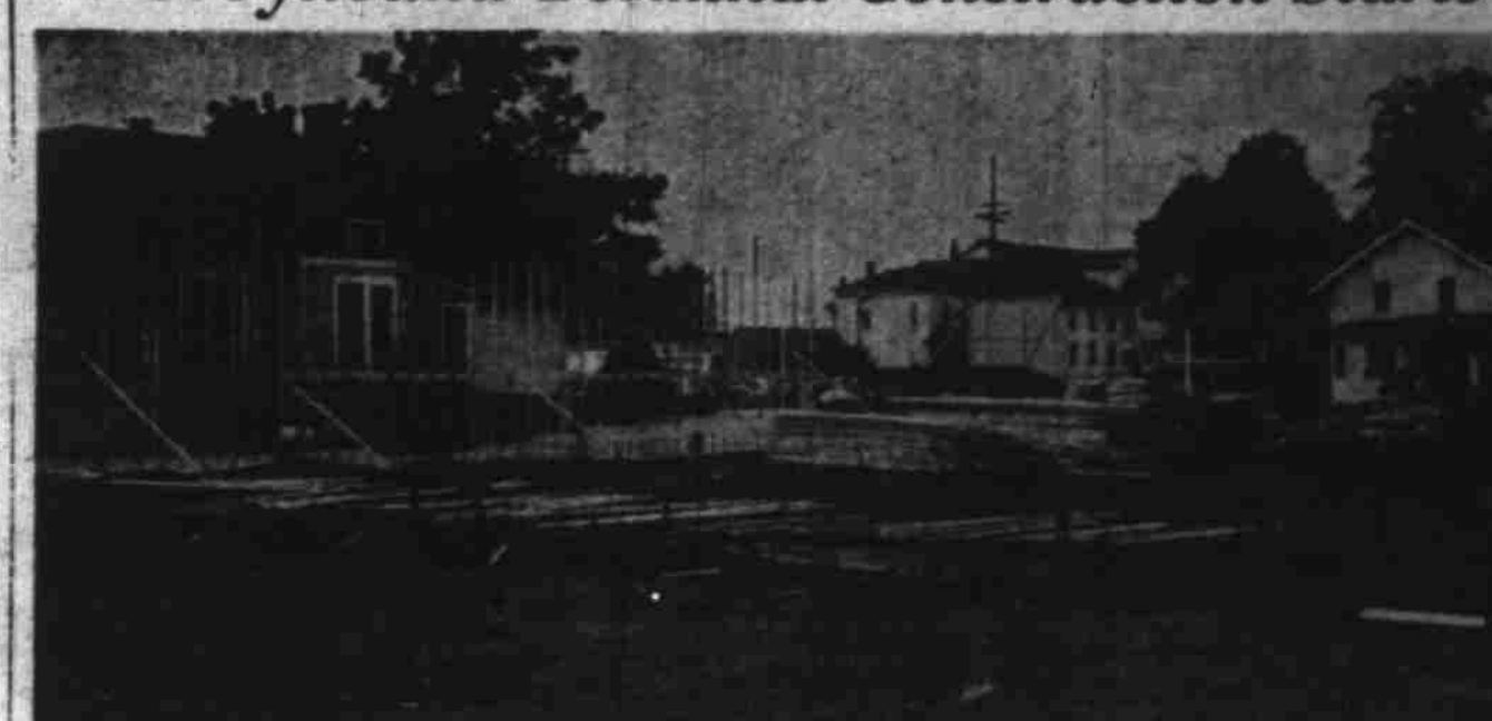
First forms for the walls of the new $112,500 Greyhound bus terminal on North Church street opposite the public school administration building are being put up this week. Photo above shows the site of the one-story reinforced concrete building, looking from the alley to North Church street. The terminal is being built by Barham Brothers, Salem contracting firm. (Photo by Don Hill Statesman staff photographer.)
