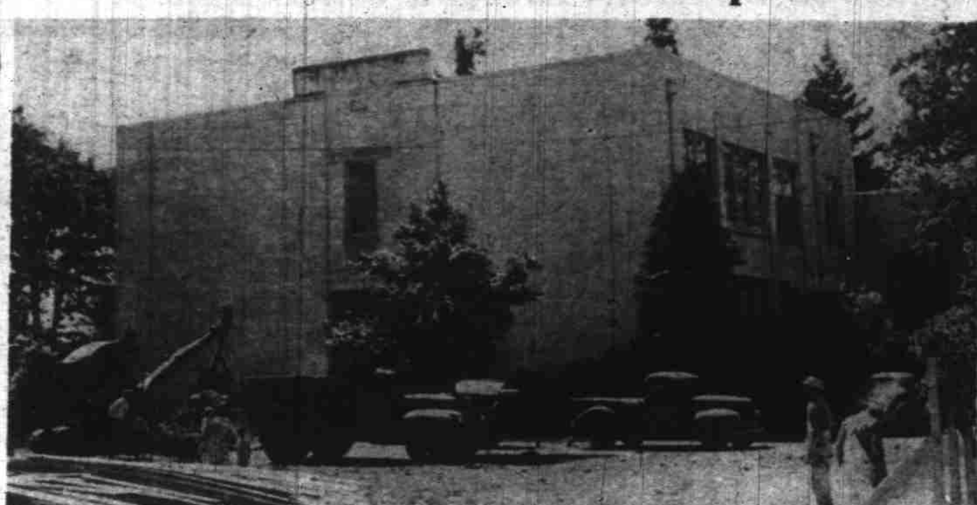
Six additional classrooms will be ready for pupils at Bush grade school next September, at the north end of the present school which is shown above. Workmen started Thursday to clear shrubbery and root out existing concrete work preparatory to beginning actual construction. The work is being done by the H. G. Carl Contracting company at a cost of $81,552.38. Carl also was successful bidder on expansion construction for West Salem and Middle Grove schools. (Photo, Don Dill, Statesman photographer).
