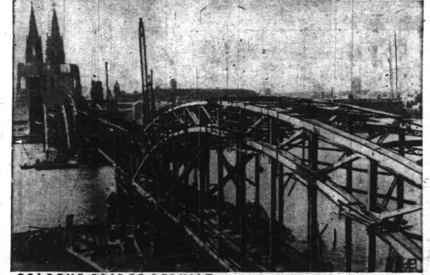
COLOGNE BRIDGE REBUILT — This is new Cathedral Bridge over Rhine River at Cologne, rebuilt to replace Hohenzollern Bridge which was blown up by retreating Germans in 1945. Parts of old bridge lie in river in background. Cologne Cathedral is at left.
