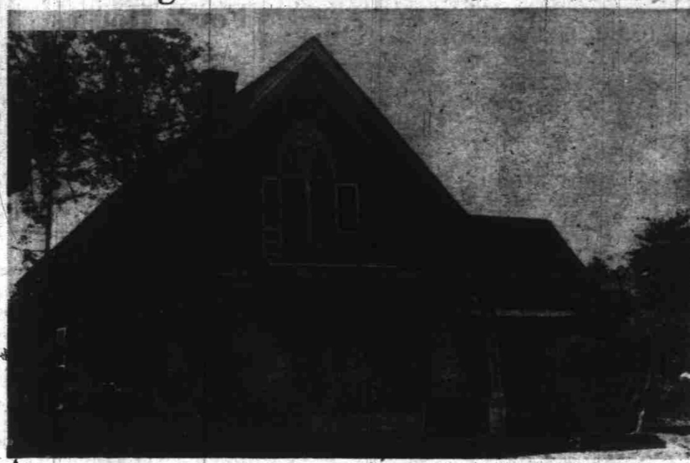
Now being wrecked to make room for a used car lot is this old Salem residence at 635 N. Commercial st. In what was once the city's finest residential area. The former William H. Byars home, it dates back nearly 80 years. (Photo by Don Dill, Statesman staff photographer).
