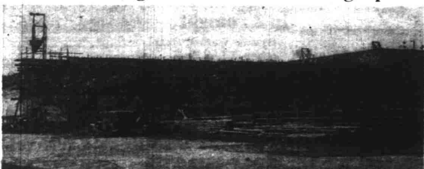
Work on the new two-story addition to the Terminal Ice and Cold Storage plant at Front and D streets is being rushed to complete the 550,000 cubic foot cold storage plant in time for this summer's growing season. Shown above is the north side of the $200,000 addition as it looks from North Commercial street. The walls are of reinforced concrete and the floors are twelve inches thick wood timbers, to aid in insulation. (Photo by Don Hill, Statesman staff photographer.)
