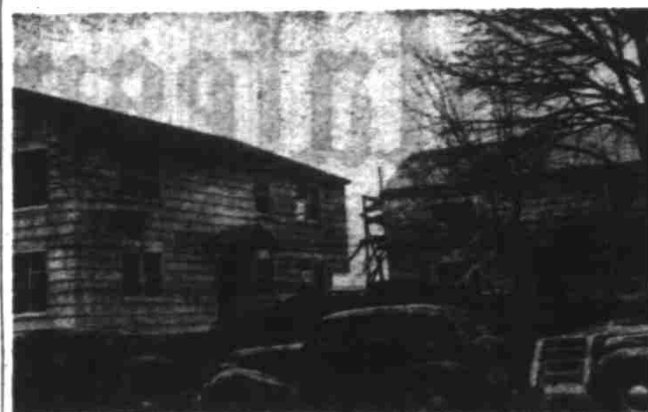
New apartment house units soon to be completed are the two shown above being constructed by J. O. Eastridge, 1955 Edgewater st. In West Salem. The two-story buildings will have eight apartments; six three-room units, and two four-room units. First apartments of the $45,000 project are to be completed sometime in April by K. I. Dodge. (West Salem contractor, and are located at 1061 Edgewater street. Photo by Don Hill, Statesman staff photographer.)
