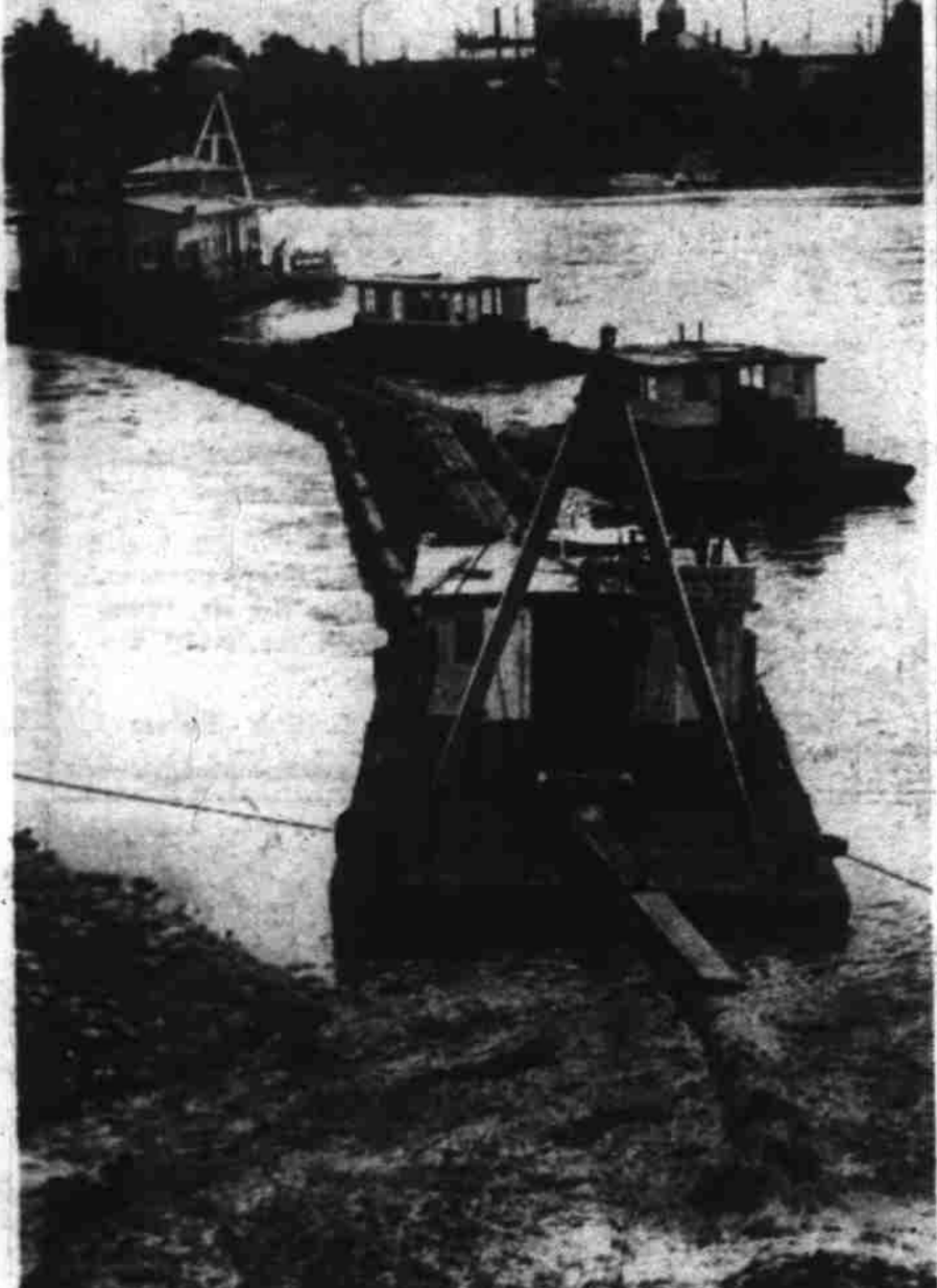
Dredging of the Willamette river in the Salem area will be completed this week by U. S. army engineer crews and the dredge Luckiamute. Gravel is sucked up by the dredge, shown in upper left corner, and piped to the river bank where the gravel and mud is discharged, shown in lower right corner. Crews cleared the West Salem bar last week, and this week will clear the Salem bar, located at the river bend north of the Union street railway bridge. (Photo by Don Dill, Statesman staff photographer.)
