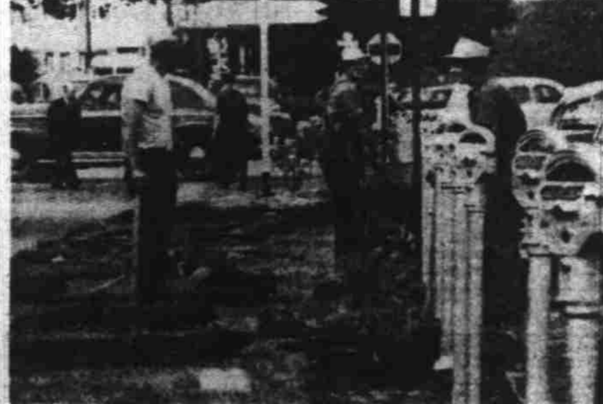
No more rose bushes blooming in the spring along the courthouse square (and snagging nylons and trousers of motorists all year long). Instead, an 18-inch concrete sidewalk, to make walking easy. The bushes now will grace Salem's city parks. Shown above at work on the project, left to right, are Bill Kessell and Joe Hovorka, both of 790 N. Church st., and H. F. Peterson, route 5, box 1042. (Photo by Don Dill, Statesman staff photographer.)
