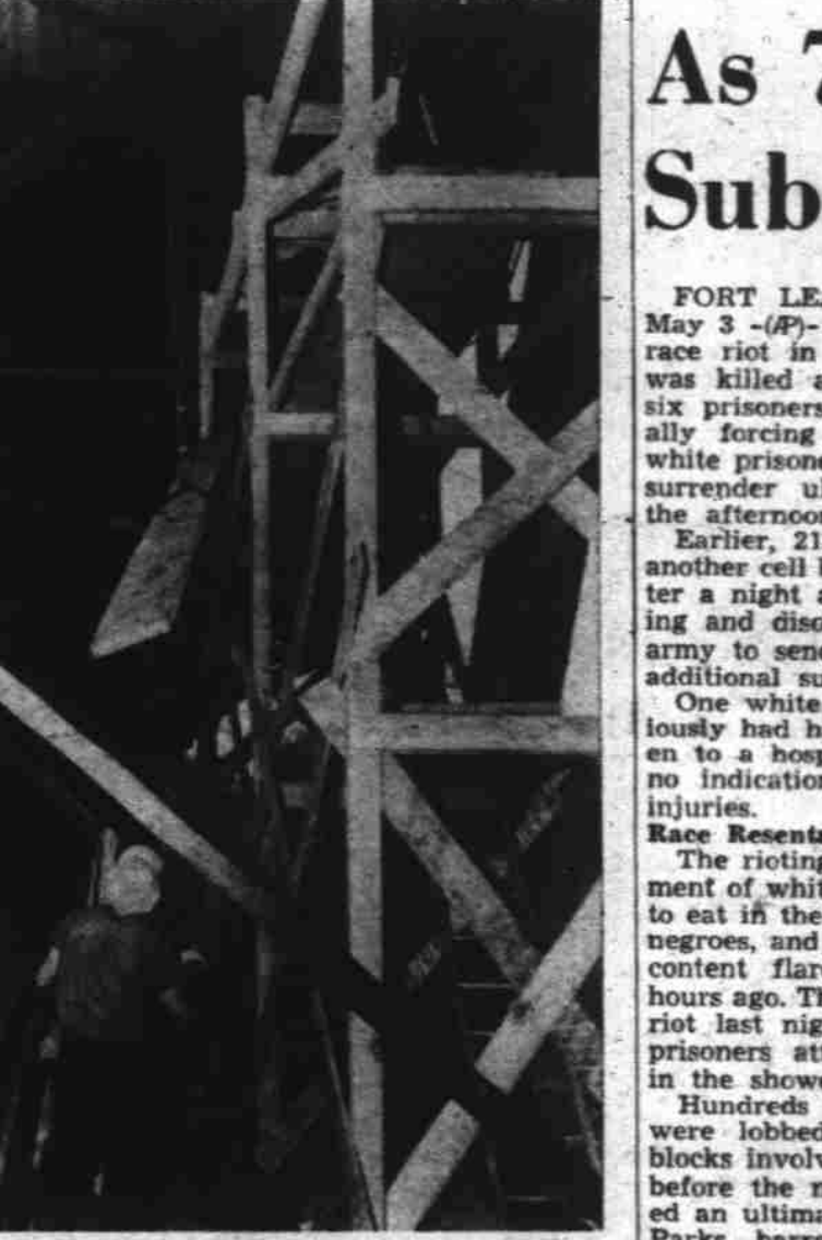
Underside of the Center street bridge linking Salem and West Salem looks like this now that workmen are putting in scaffolding preparatory to installing a pipeline to boost West Salem's water supply and alleviate its annual drought. Some 2,300 feet of eight-inch pipe will connect the two water systems. 970 feet of the pipe to be strung just underneath the bridge. Contractor G. R. Boatwright expects the part of the installation across the river to be completed in about 10 days. (Statesman photo by Don Dill, staff photographer.)
