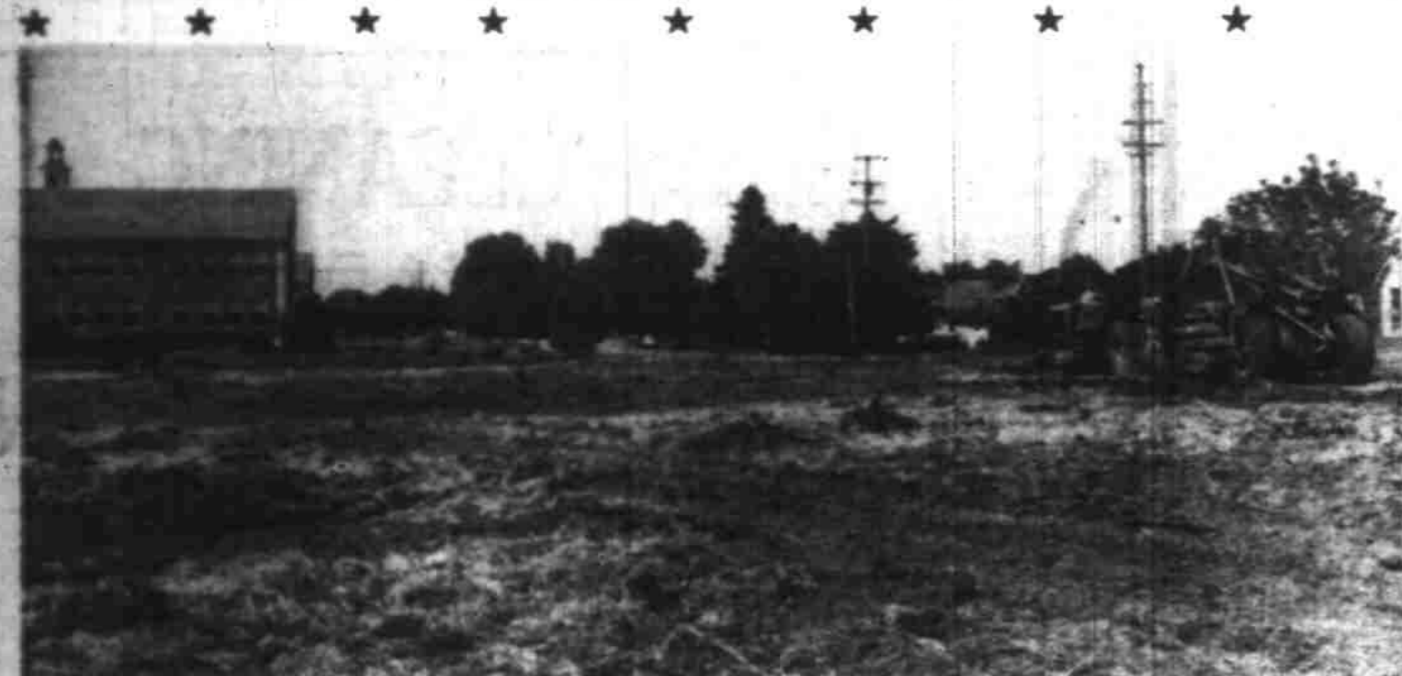
PROOF: If you still doubt that one day soon Salem high's new football stadium will blossom on part of what is now Olinger field, take a look at D. H. Hooper (above) pulling a 16-yard carryall for the C. T. Malcolm construction company during ground-breaking chores this week. The photo was taken while looking toward the school buildings from the Olinger swimming pool and park area. Trees, shrubs and assorted junk felt the leveling machinery. The Vikes hope to trot onto their new field in the fall of next year. (Bill Scott photo).
