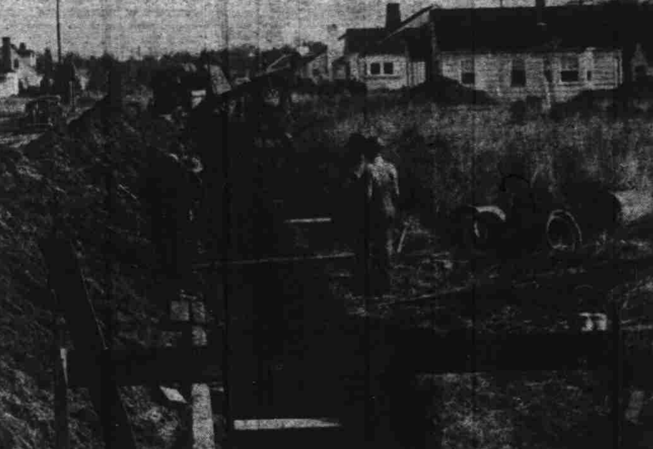
First major postwar public work in Salem, the $10,000 Rosedale relief sewer is under construction today. This picture, taken near the intersection of Baker and Norway streets by a Statesman photographer, shows a crew, short of needed men, lowering 18-inch concrete tile into position. Friday's rain served notice that there can be little delay if the project is to be completed in time to save basements of the Rosedale district from floods they have experienced the past several winters.
