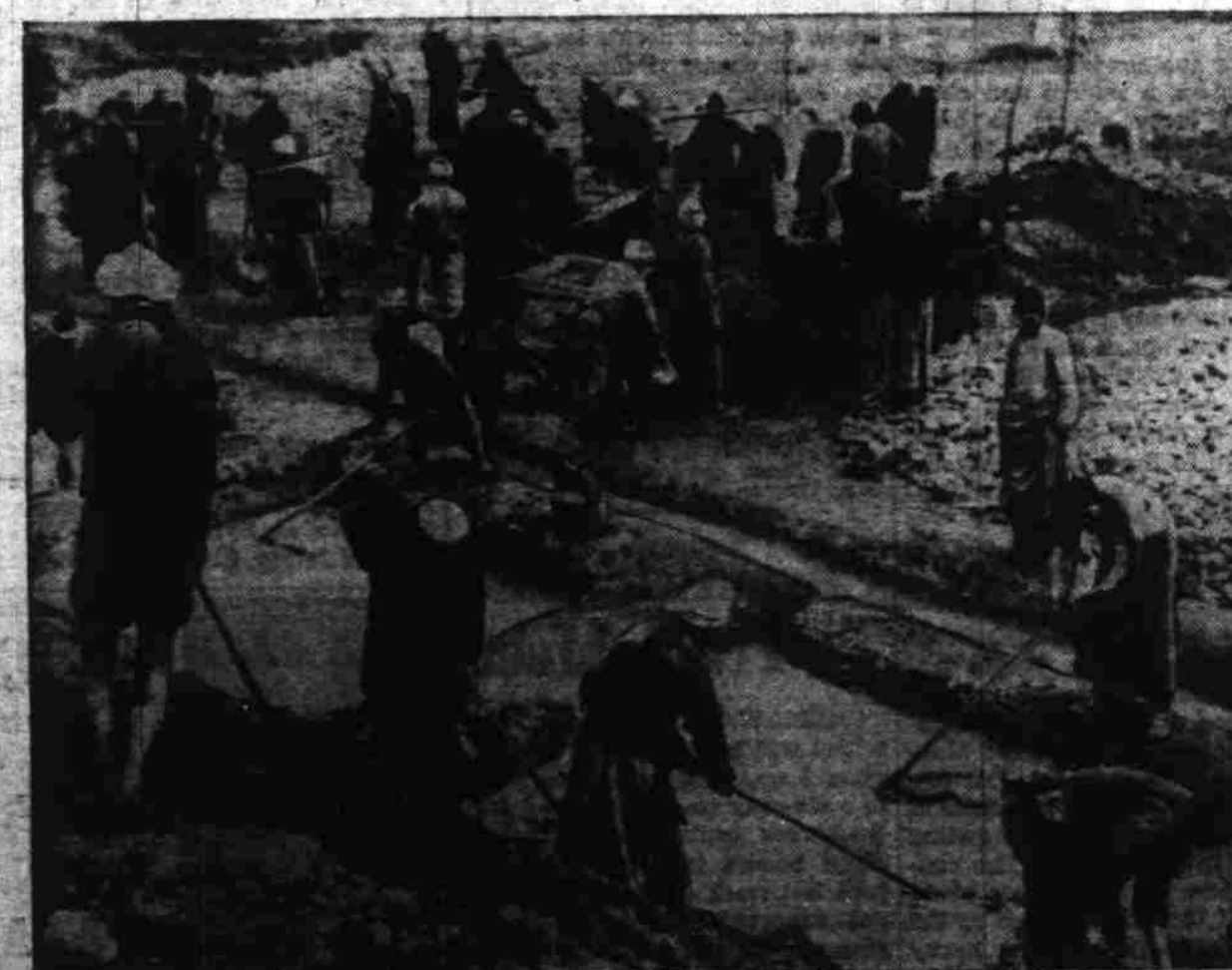
CHINESE BUILD RUNWAY —Using age-old equipment more familiar to them than modern tools which are not available, Chinese laborers prepare material for an airfield runway.
