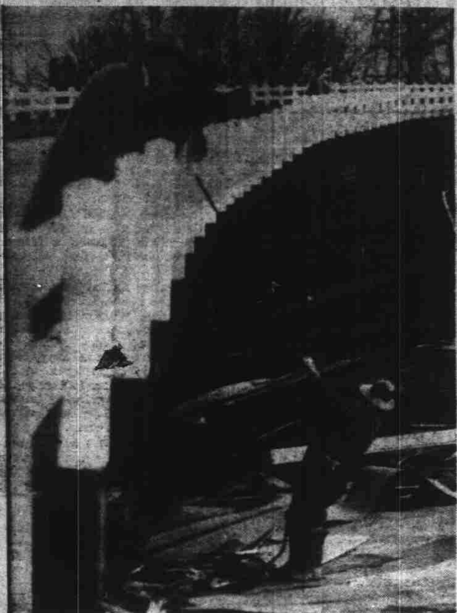
F. W. "Jerry" Farrar, district maintenance superintendent for the highway department, examine wreckage of the Mellow Moon skating rink, jammed against the west approach of the inter-county bridge, before ordering workers to tear it up to take off pressure. Looking down and assisting are E. G. Ricketts of the state highway department; J. M. Hartley, bridge guard; H. A. Belensifer of the telephone company; Capt. Walter Lansing of the state police, and Lloyd Edgell.—Statesman photo.
