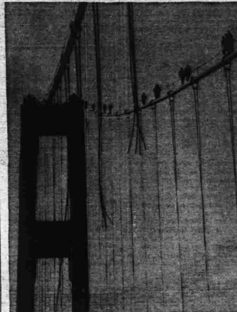
Men dismantling the wrecked Narrows bridge at Tacoma, Wash., for scrap, walk along suspension cable high above the water. The cables of the bridge are expected to yield 3000 tons of steel.—Associated Press Telegram.
