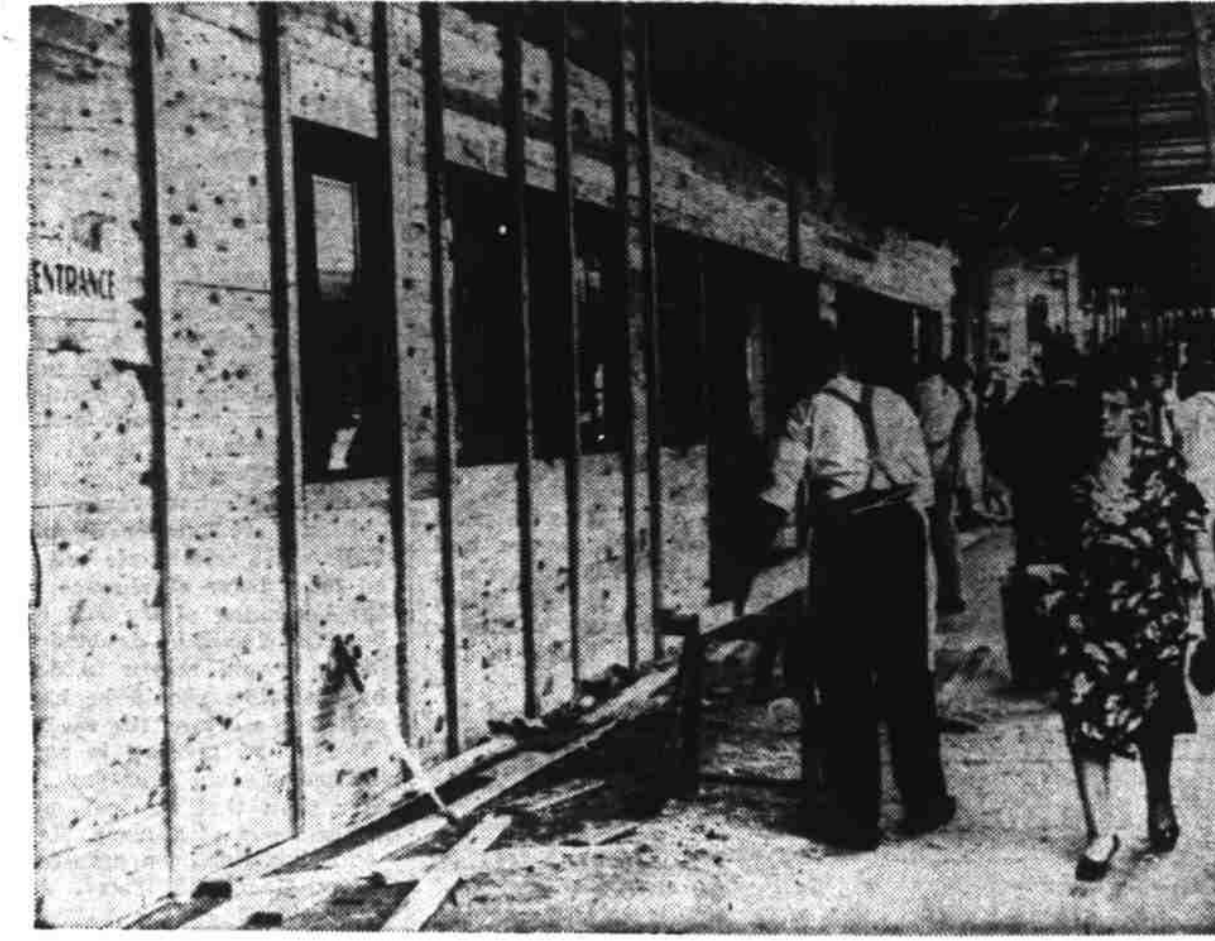
The menace of flying glass from bomb blasts is being anticipated in Sydney, Australia. This firm with a series of show windows, is removing all glass, except for small panels, and replacing the panels with heavy plywood.
