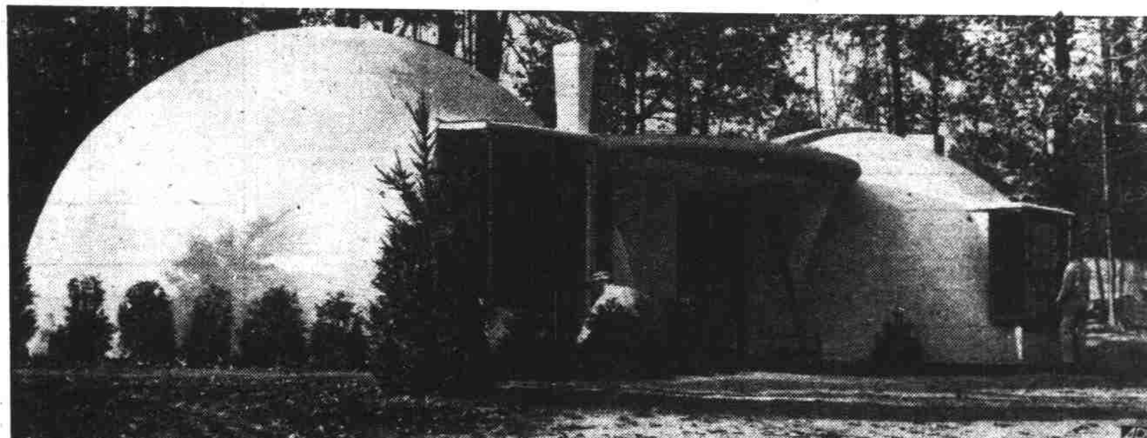
NECESSITY MOTHERS A NEW ONE —To satisfy demands for simple, inexpensive homes in defense production centers, this experimental igloo-type house was built in Fairfax county, Va., workmen spraying concrete mixture onto inflated rubber forms.
