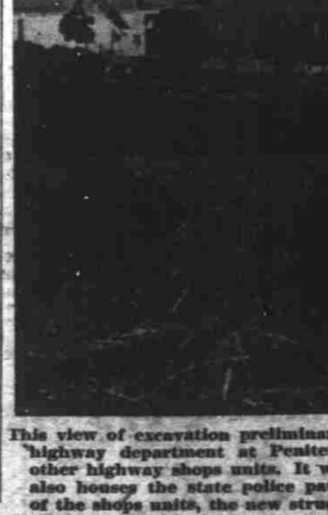
This view of excavation preliminary to erection of an $80,000 laboratory-office building for the state highway department at Pentecostal and Airport roads gives an idea of its location with respect to other highway shops units. It will be adjacent to the highway sign shops building, at right, which also houses the state police patrol office and the highway traffic engineering division. Unlike other of the shops units, the new structure will be of reinforced concrete construction.—Statesman photo.
