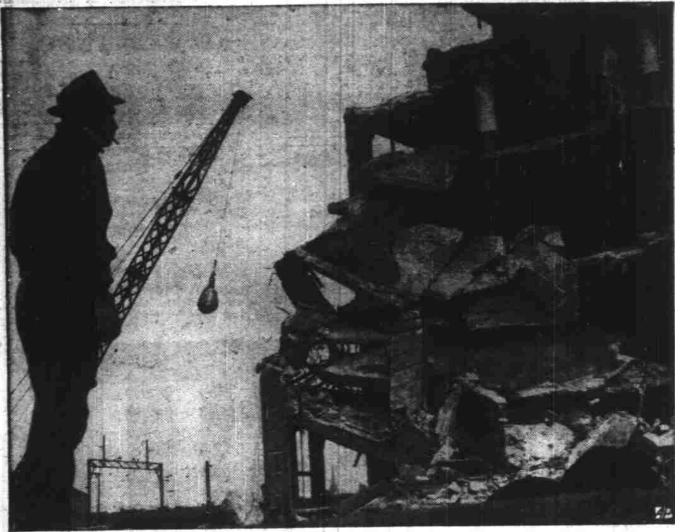
LOOK OUT BELOW! —An eight-story concrete building comes tumbling down in Philadelphia under the heavy blows of a swinging steel ball. Engineers used the ball, hung from a 70-foot crane boom and swung like a clock's pendulum, to raze the building for a new housing project. In this "angle" shot, a workman watches results.
