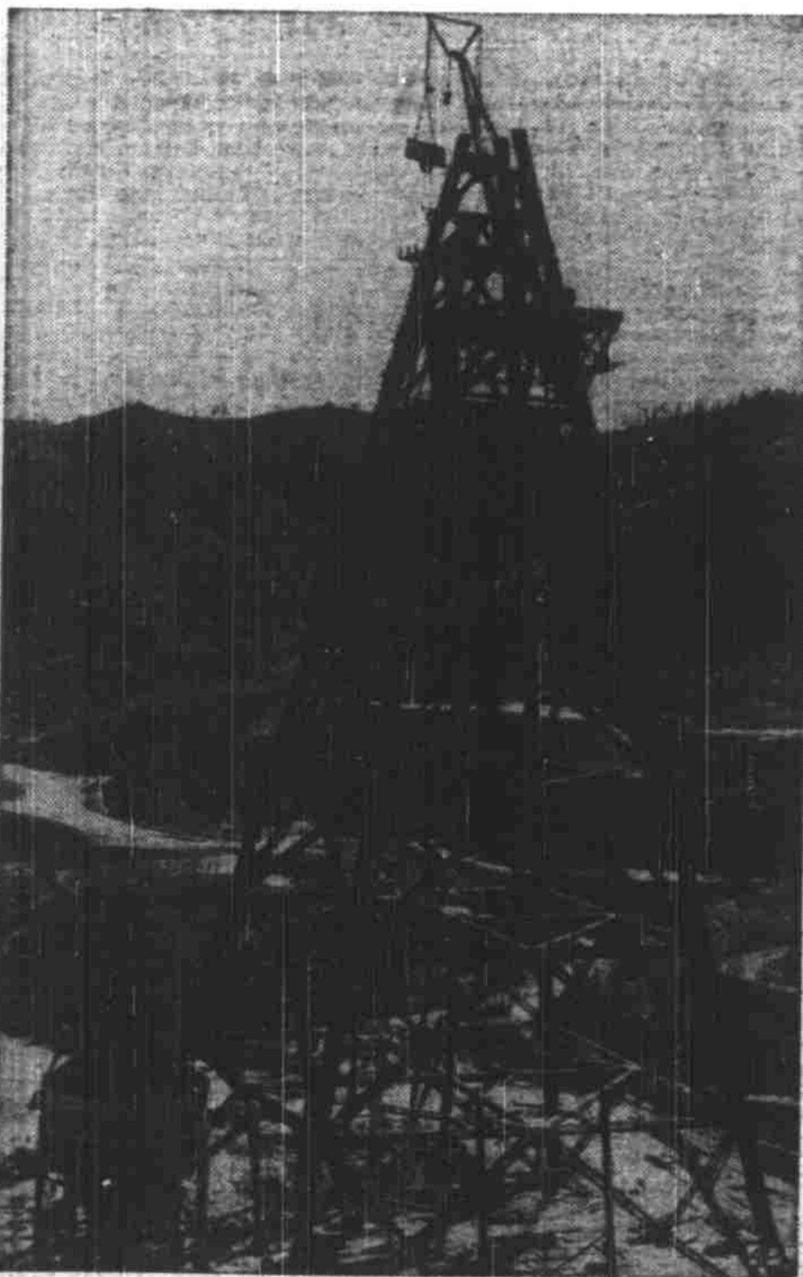
DESERT SKYSCRAPER —From this 460-foot tower will suspend the seven cables anchored at key points surrounding Shasta dam, California, thus providing seven inclines over which concrete-bearing buckets will glide. Shasta dam is being built by the U. S. Bureau of Reclamation to control the water and power of the Sacramento and San Juan rivers.
