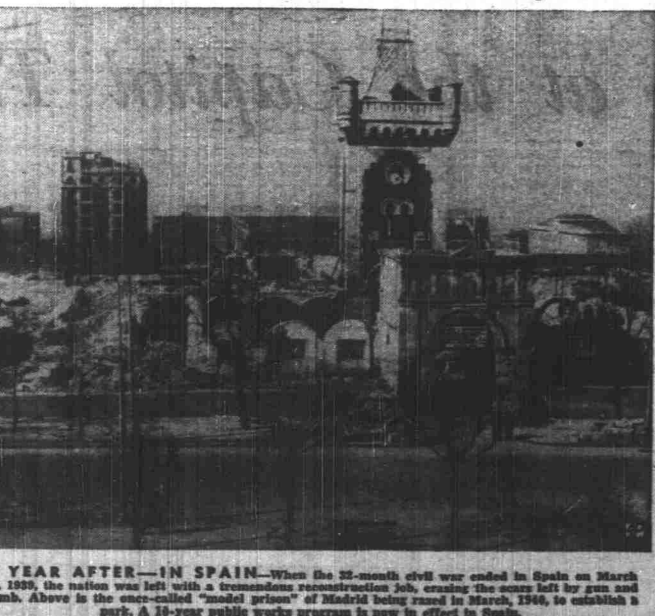
A YEAR AFTER—IN SPAIN—When the 22-month civil war ended in Spain on March 28, 1939, the nation was left with a tremendous reconstruction job, craning the scars left by gun and bomb. Above is the once-called "model prison" of Madrid being raised in March, 1946, to establish a part. A 10-year public works program is now in effect in Spain.
