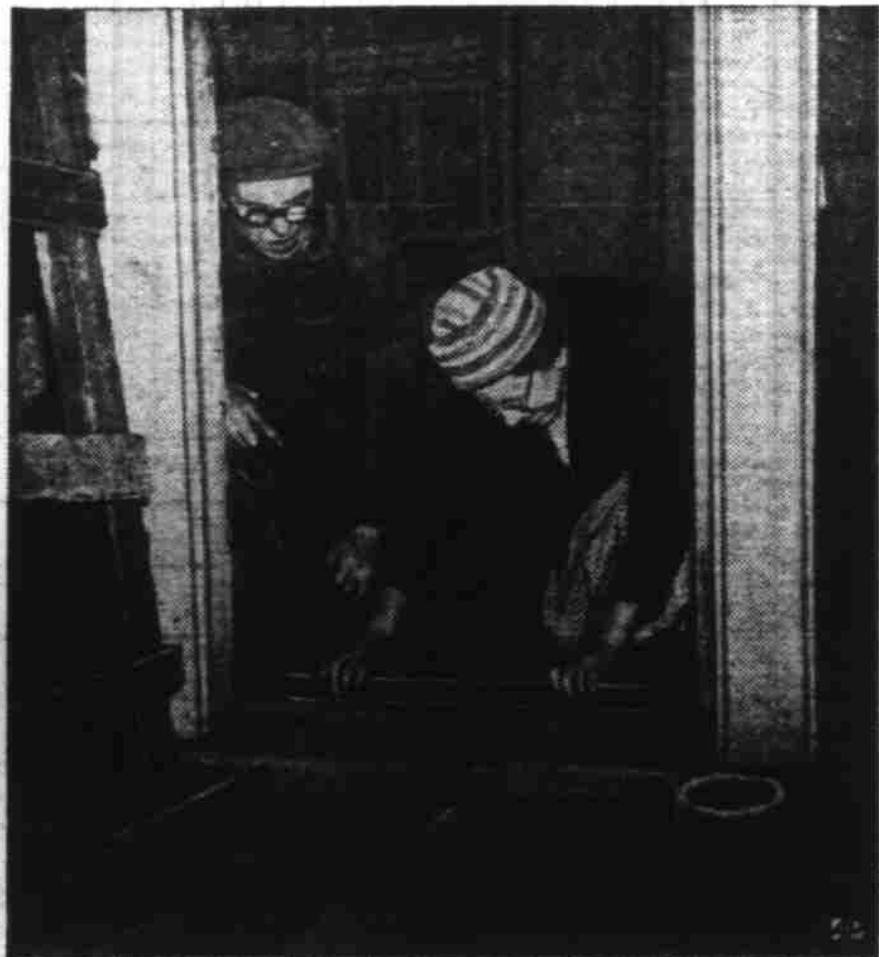
HELPING HANDS —To make sure that things are "on the level," Mrs. Mary Grove checks up on doorway in a two-story addition being built by her husband, Robert (above), who's almost totally blind. They live in Wilkins Twp., Pa.
