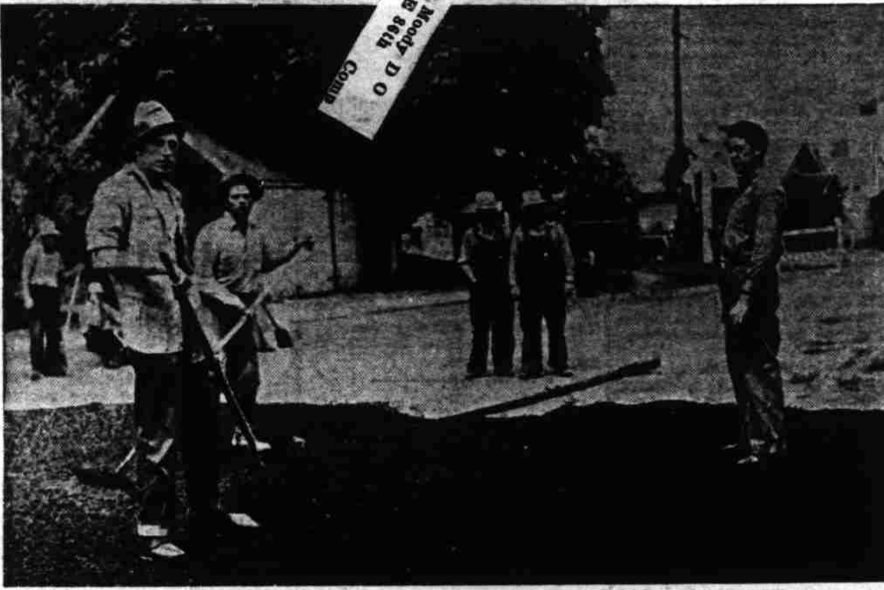
West Salem, the little city with courage enough to pave all its streets at once, saw the surfacing program begin materializing yesterday as WPA workmen, shown above, spread the first hot, bituminous material on the subgrade of Gerth avenue between Edgewater street and the railroad. Five miles of paving, 10 miles of curb-laying will be done before the project is finished. The city's share of the cost will be around $50,000.
