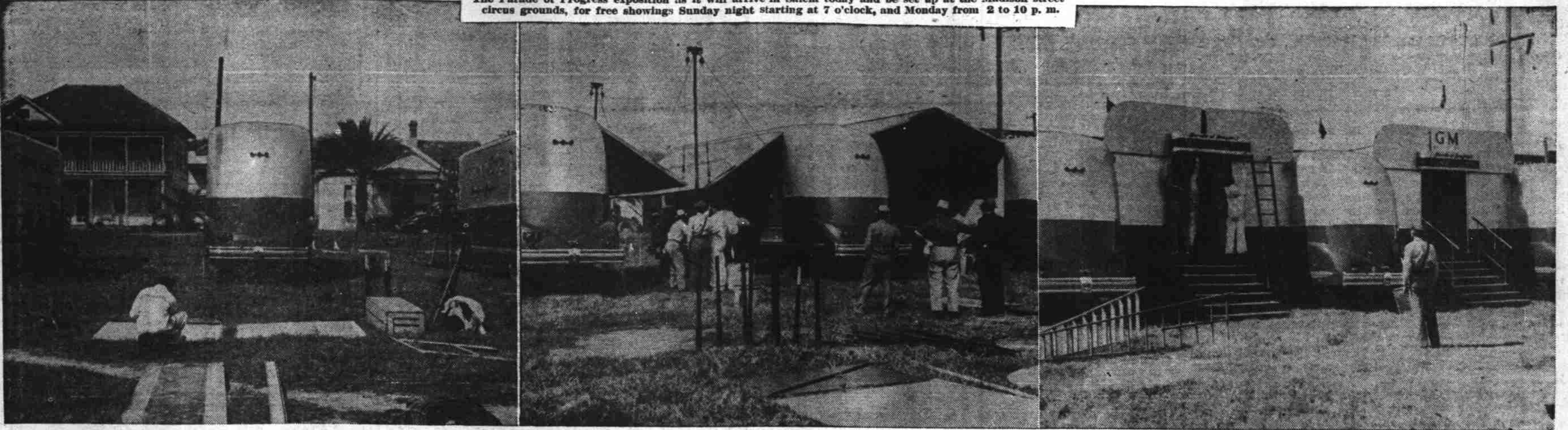
Red and silver "Streamliners" of General Motors are driven onto the show grounds. They must be "spotted" and leveled, then spaced exactly 14 feet apart. An inch off level makes erection difficult.
