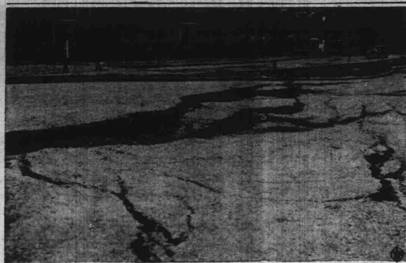
Web of cracks in $500,000 project
