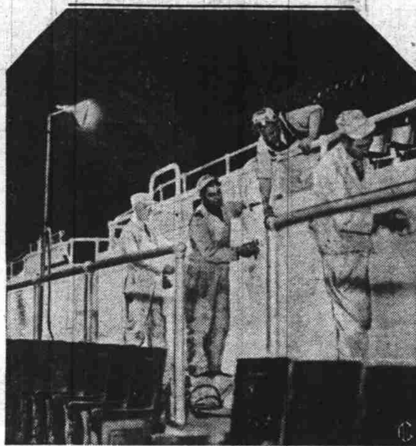
New flooring and extensive repairs to the Cleveland Public auditorium were rushed to completion by a small army of workmen in preparation for the 1936 Republican convention opening June 9.
