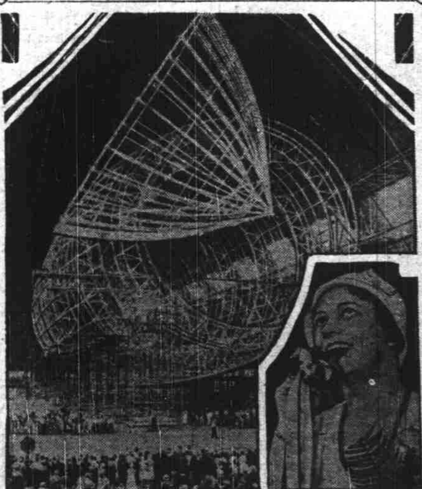
Here's the scene inside the giant hangar at Akron, Ohio, as the nose of the new dirigible U. S. S. Macon, sister ship of the Akron, was set in place. Elaborate ceremonies marked the step towards the completion of the United States new sky queen, many distinguished visitors from the Georgia city for which the craft is named participating in the event. Inset: Miss Susan Myrick, of Macon, Ga., who blew the whistle which signaled the beginning of the placing of the bow in position.
