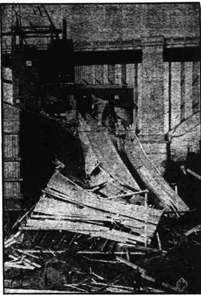
View of the huge coal storage shed of the McNulty Brothers Coal Co., New York, after it collapsed, sending 900 tons of coal down upon seven men working beneath the structure, who were buried alive with no chance to escape. Police and fire department rescue squads with hand and steam shovels worked desperately to uncover the men in their tombs under the mountain of coal.
