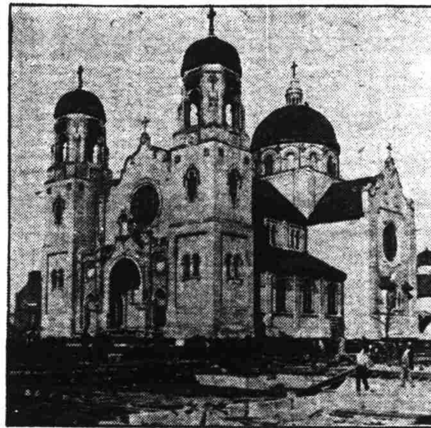
MOVED ACROSS STREET, this Church of Our Lady Loudres, Chicago, is none the worse. The undertaking required 200 workmen, four stationary tractors, 50,000 feet of steel cable, 3,000 steel rollers, 4,000 jacks and 50,000 feet of timber.
