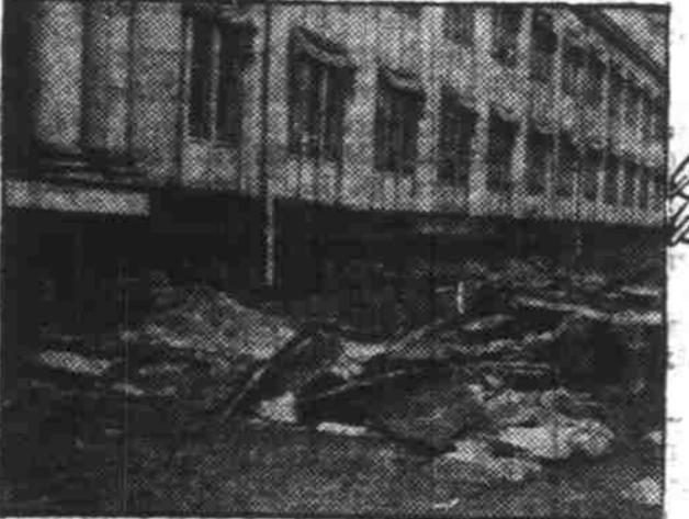
LEFT—$25,000 DAMAGE DONE BY TERMITES TO THIS TEMPORARY WAR STRUCTURE. MATURE SOLDIER TYPE OF WHITE ANT. (RIGHT) WINGED FORM TERMITE. RIGHT—TEST SHACK IN CANAL ZONE BUILT OF CHEMICALLY TREATED WOOD.
