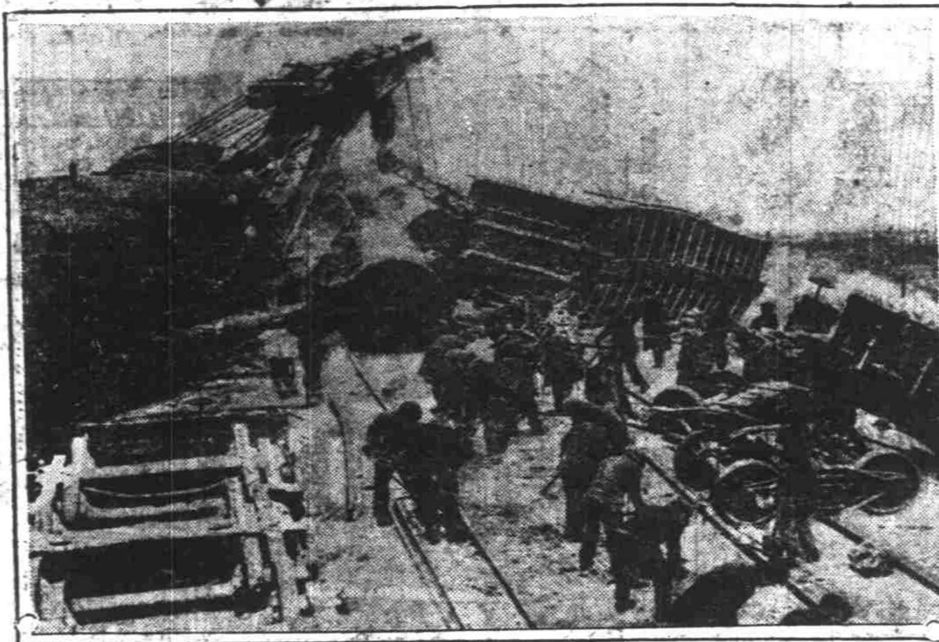
Blinding snow storm that was raging at the time is blamed for the wreck of 28 cars of a 90-car Milwaukee & St. Paul R. R., near Milwaukee. Other trains were held up for some hours. Photo shows wrecking crews at work.
