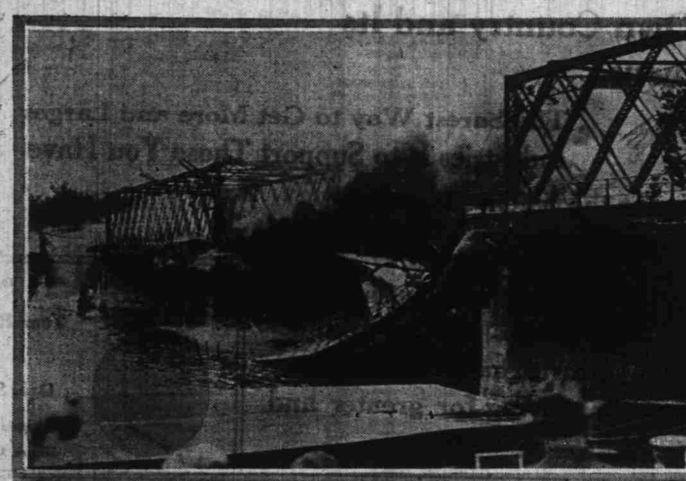
View of the fire wrecking the big North End Bridge, spanning the Connecticut River between the city of Springfield and the town of West Springfield, Mass. The intense heat quickly buckled and wrecked the steel framework. The bridge was the only means of trolley communication between Springfield, West Springfield, Westfield, and Holyoke, while an old covered wooden bridge, scarcely safe, is all that is left for auto and horse or foot traffic. The fire severed a gas main, trunk line telephone cable, a large water main, and several trunk line telegraph cables. The town of West Springfield, dependent on Springfield for lighting current, was shrouded in darkness. It is estimated the total loss will approach a million dollars.
