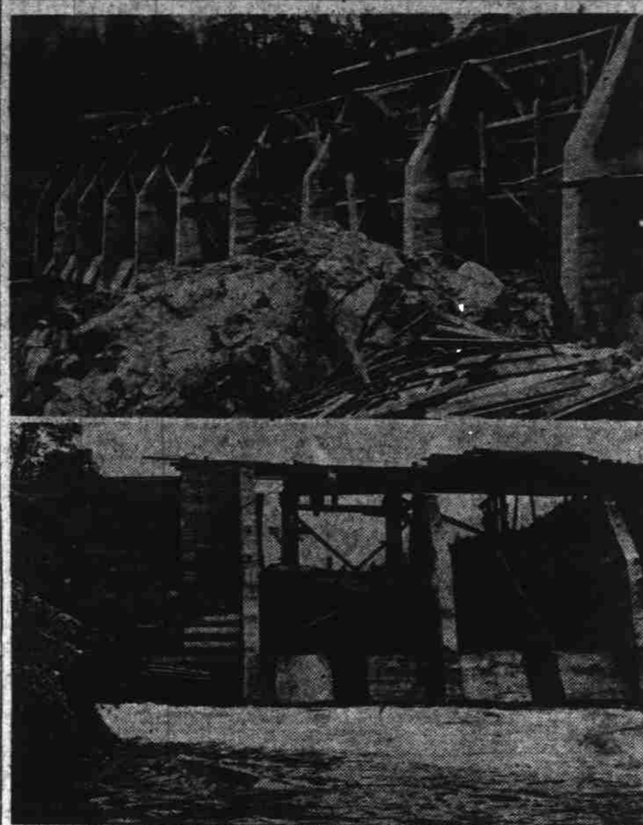
Above—Savage Rapids Irrigation dam. Below—Power house, where water will be pumped to high line ditches.
