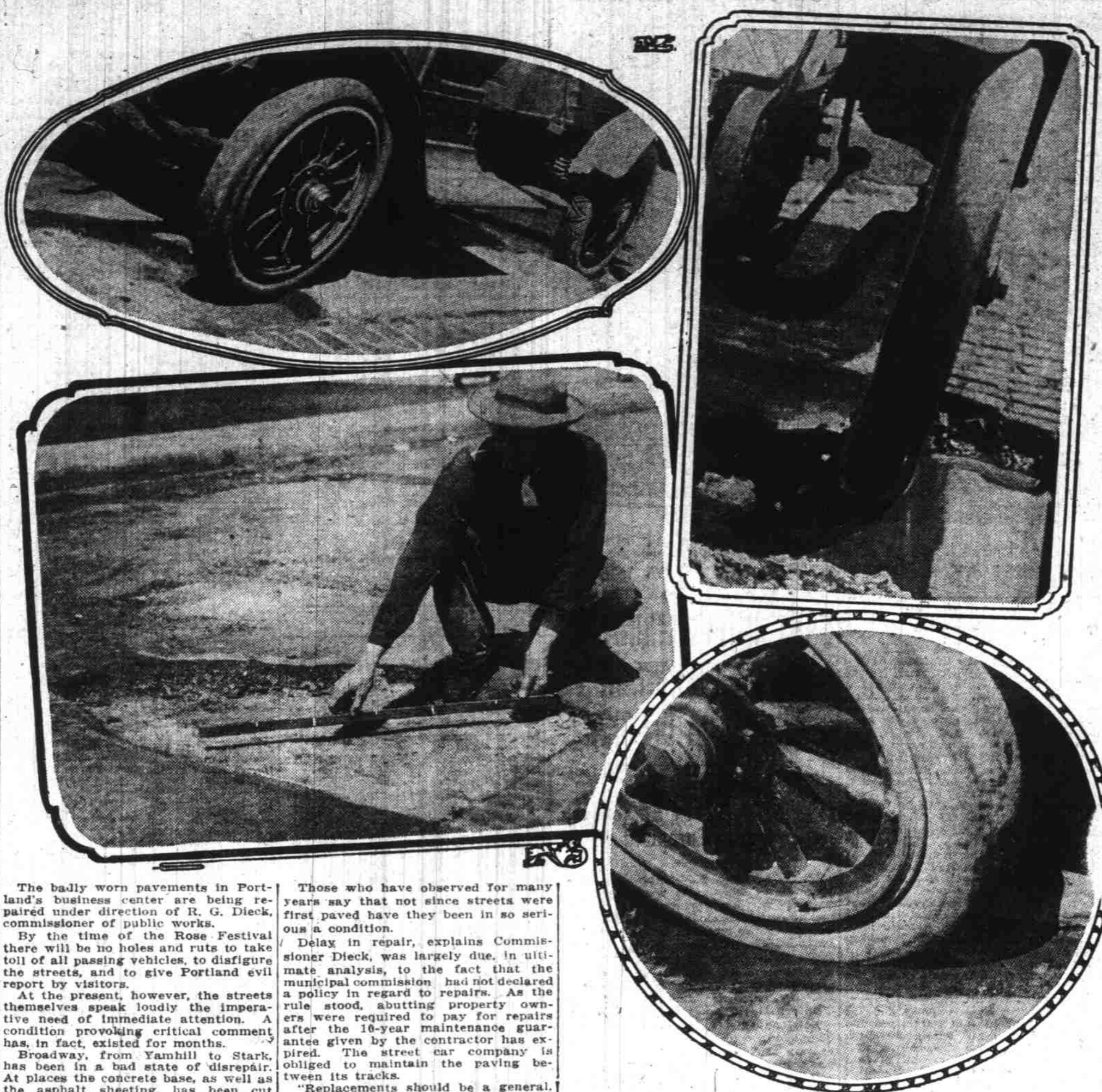
Top, left to right—Rut on Broadway between Washington and Alder. Water-filled hole, Stark near Broadway. Bottom, left to right—Man measuring width of hole on Broadway. Corner of Stark and Broadway. These views are typical of many other paved streets in Portland which will be repaired this spring.
